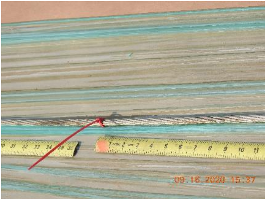
Figure 7: Residue on subject conductor.
