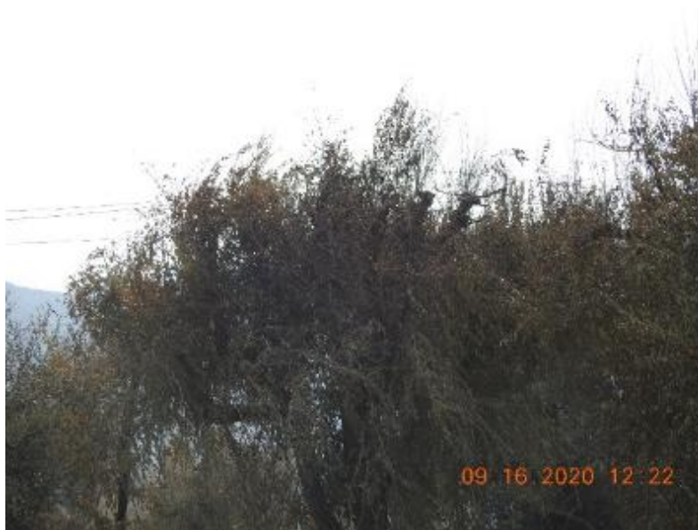
Figure 2: Three fallen conductors between the two H-frame structures resting on the trees below.
