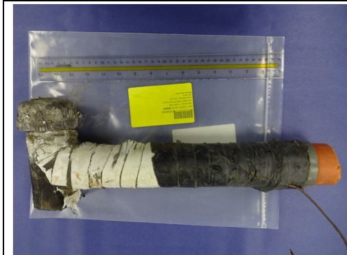
Figure 3. Photograph of Mueller Tee after removal from scene. 3
