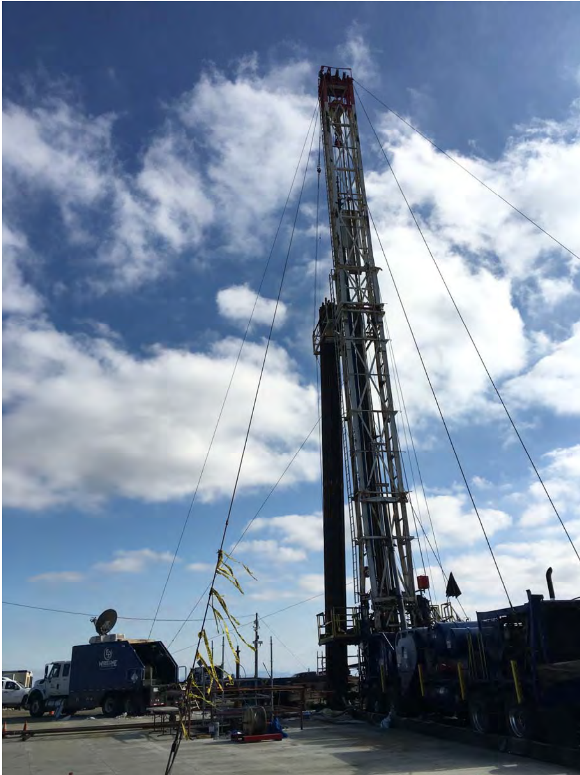
Figure 1. Ensign #334 on Well SS-25A in May 2017. Well SS-25 is located in the foreground between the rig and logging truck.
