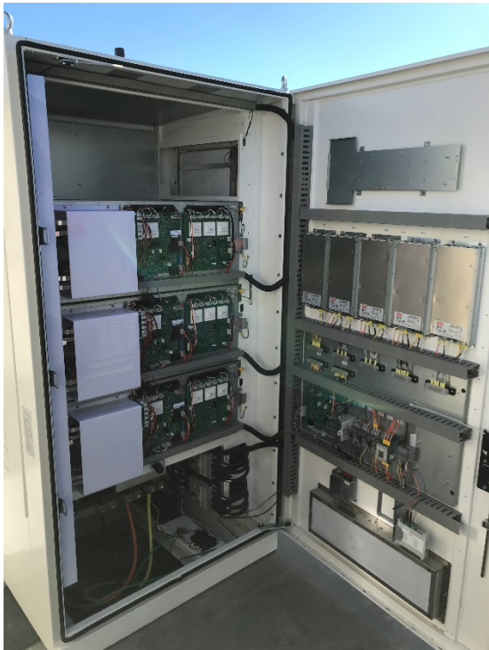
Image 13: BTC 150 kW power cabinet interior.
