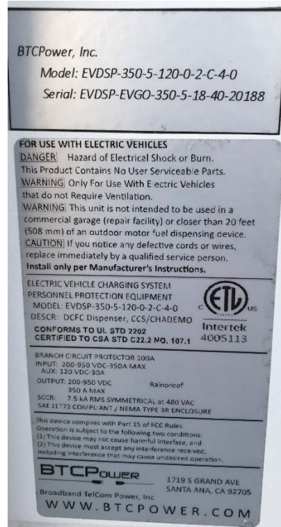
Image 10: BTC 150 kW charger nameplate.
