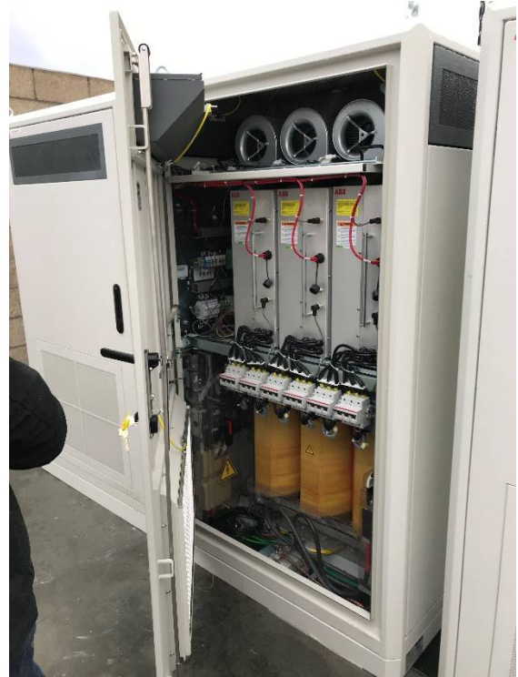
Image 6: ABB 175 kW power cabinet interior.
