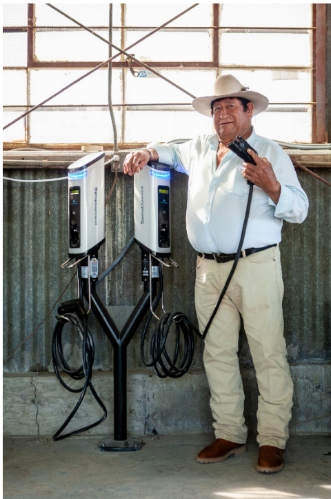
Image 3: Community Member with Level 2 charger installed at the Huron headquarters
