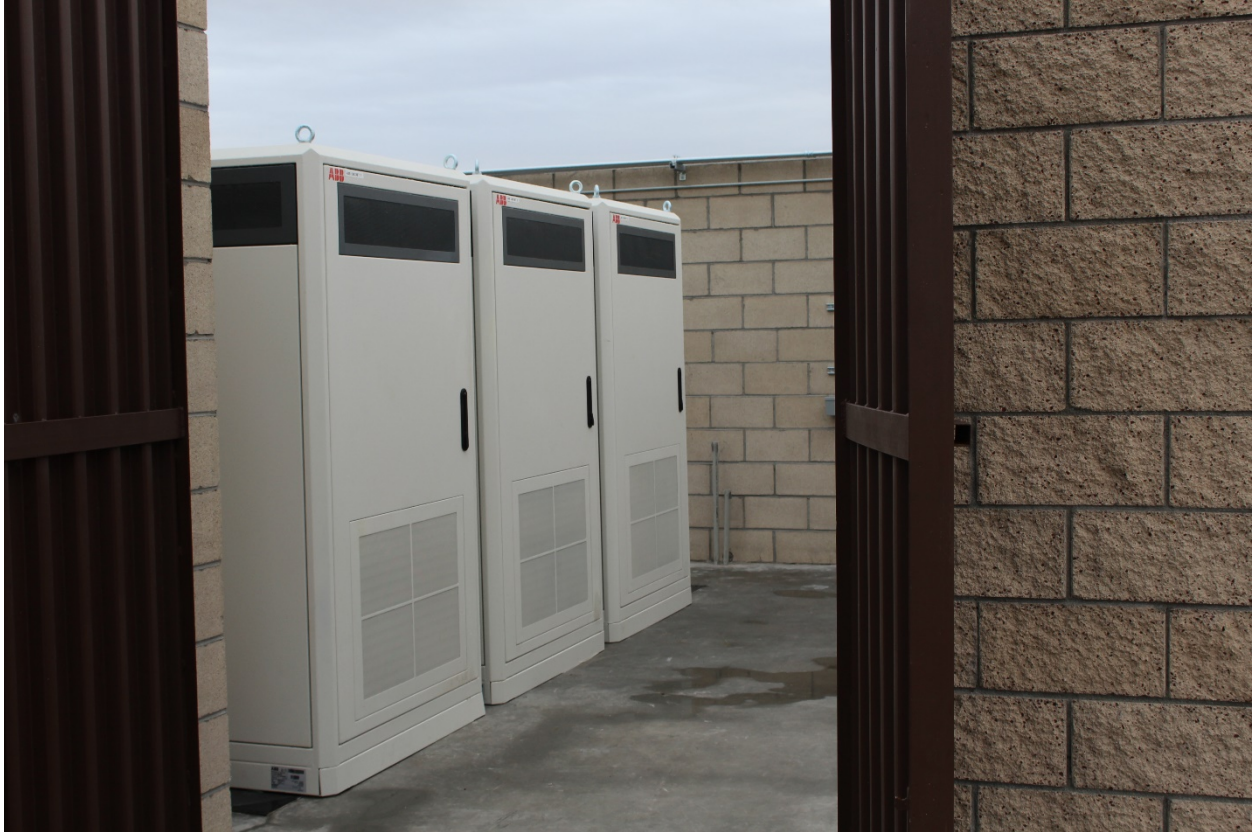
Image 4: ABB power cabinets. 1 cabinet feeds the 175 kW charger, 2 cabinets feed the 350 kW charger.
