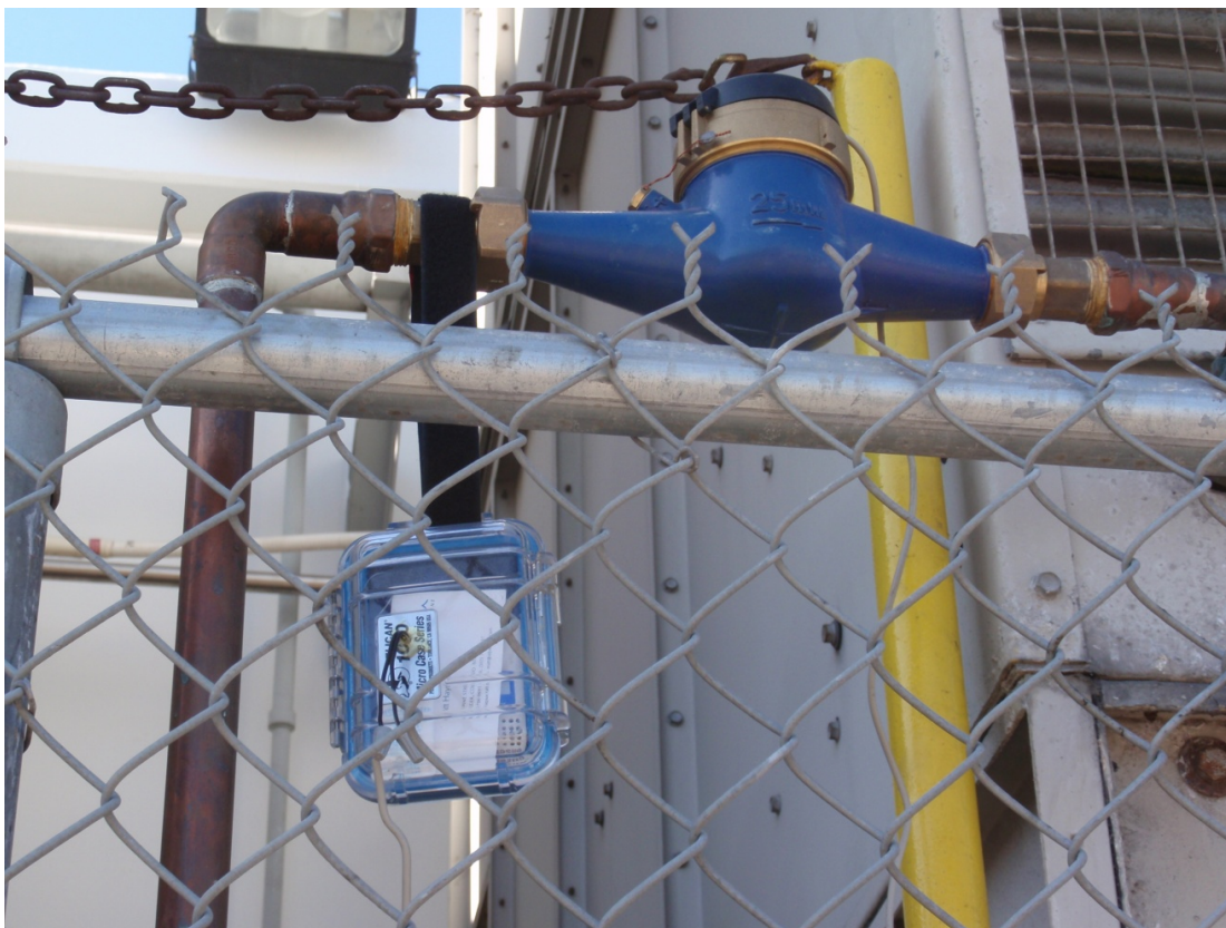
Figure 20: Photo of Water Meter and Data Logger (in case) on Water Supply Line
