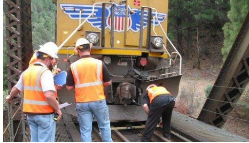
UPRR work train locomotives, Maintenance of Way workers and CPUC Track railroad safety inspectors testing track geometry including gage, cross level and elevation under load near POD at Gibson derailment site.
