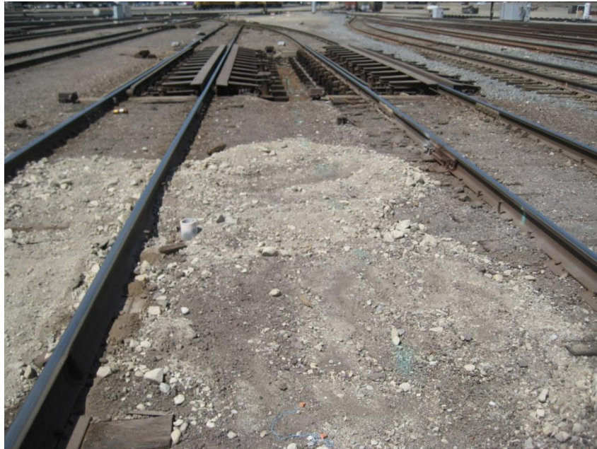
Rough and Uneven Walkway with Substantial Debris – GO 118 Defect UP West Colton Yard
