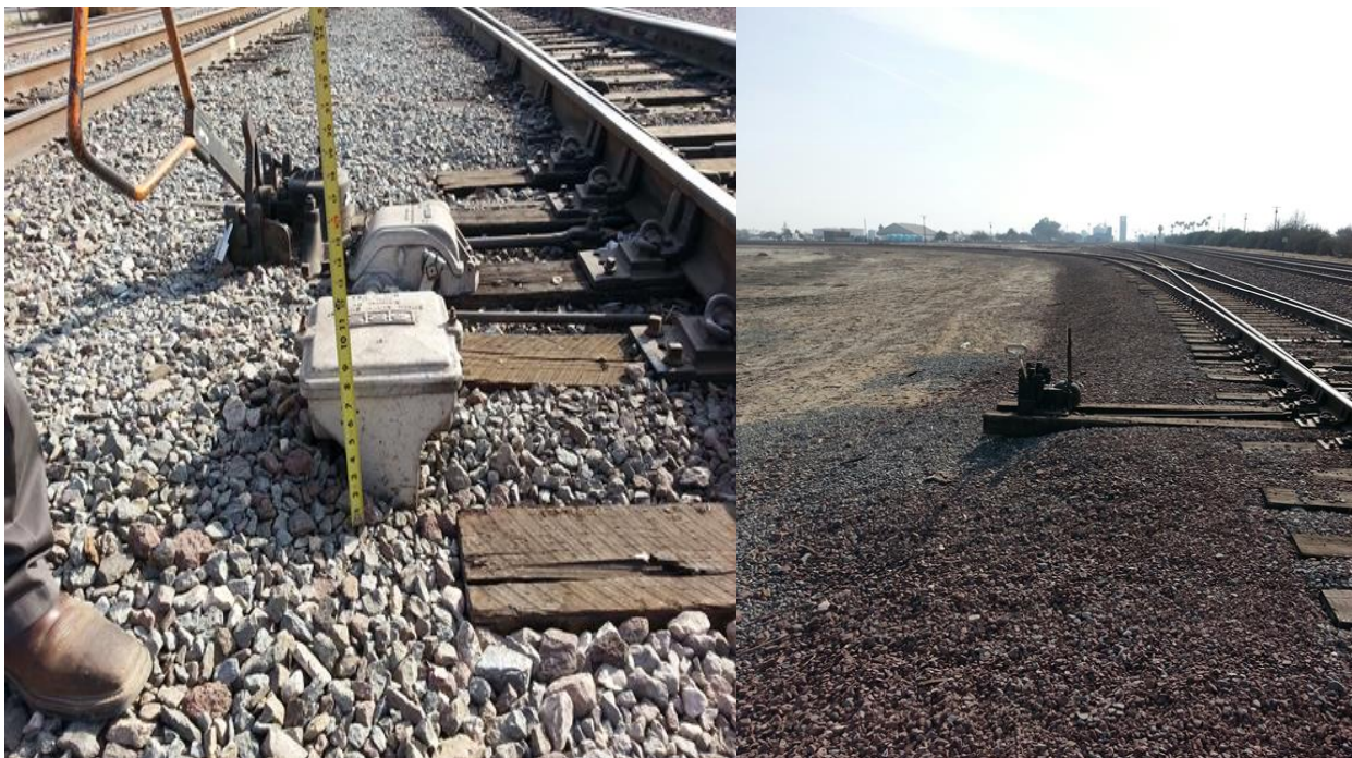
Photo to the left is a junction box that is in the walkway creating a tripping hazard for trainmen. The top of the box should be level with the walkway. Photo to the right shows a steep slope to the left of the switch. There is no safe place for a trainman to stand while lining the switch. A three foot level walkway is required behind the switch stand.
