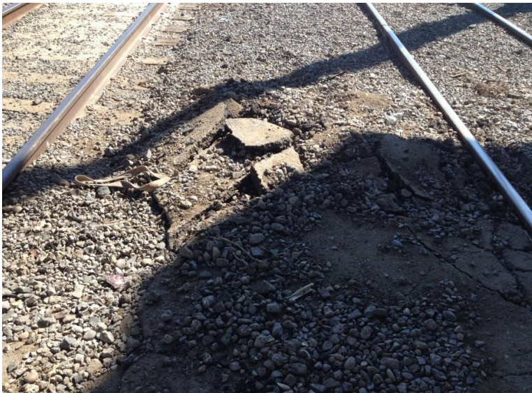
Uneven walkway surface can lead to serious injury of crew members working alongside moving equipment, Such conditions do not comply with State General Order 118-A
