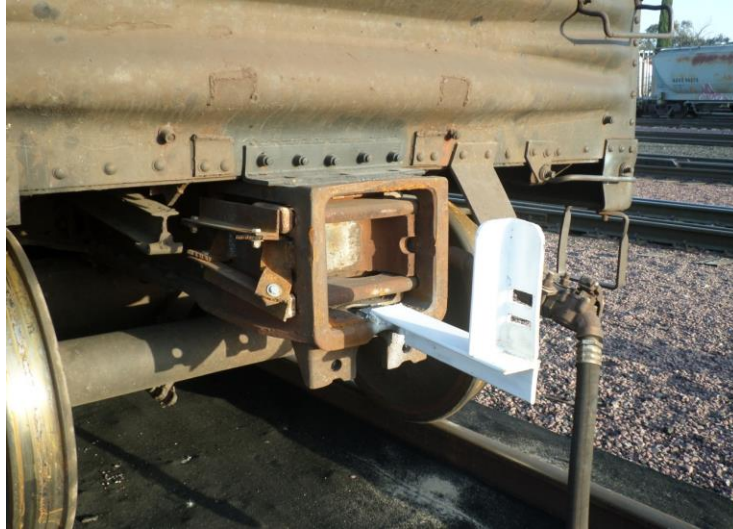
Defective car with missing coupler
