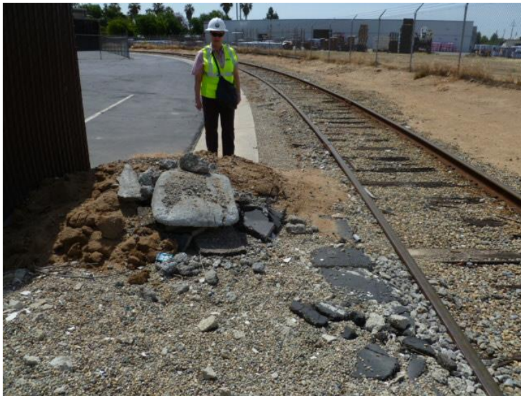
This pile of debris in the walkway of an industrial lead track on the Clovis Branch is a GO 118-A defect. The debris poses a hazard to trainmen either tripping, or fouling the track and possibly being struck by moving equipment while trying to get around the pile of dirt, asphalt and concrete.
