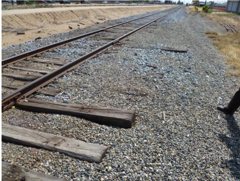
Long ties extend into the walkway, posing a tripping hazard, remnants of a track that was removed. This condition does not comply with GO 118-A.
