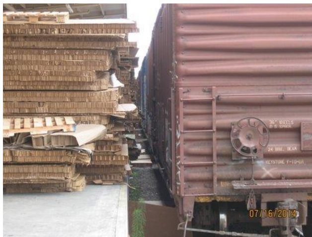
Inspection of facility in Benicia revealed two State General Order defects, both unsafe for railroad workers: One is a clearance issue, the other a tripping hazard due to obstacles left on the dock and in the walkway
