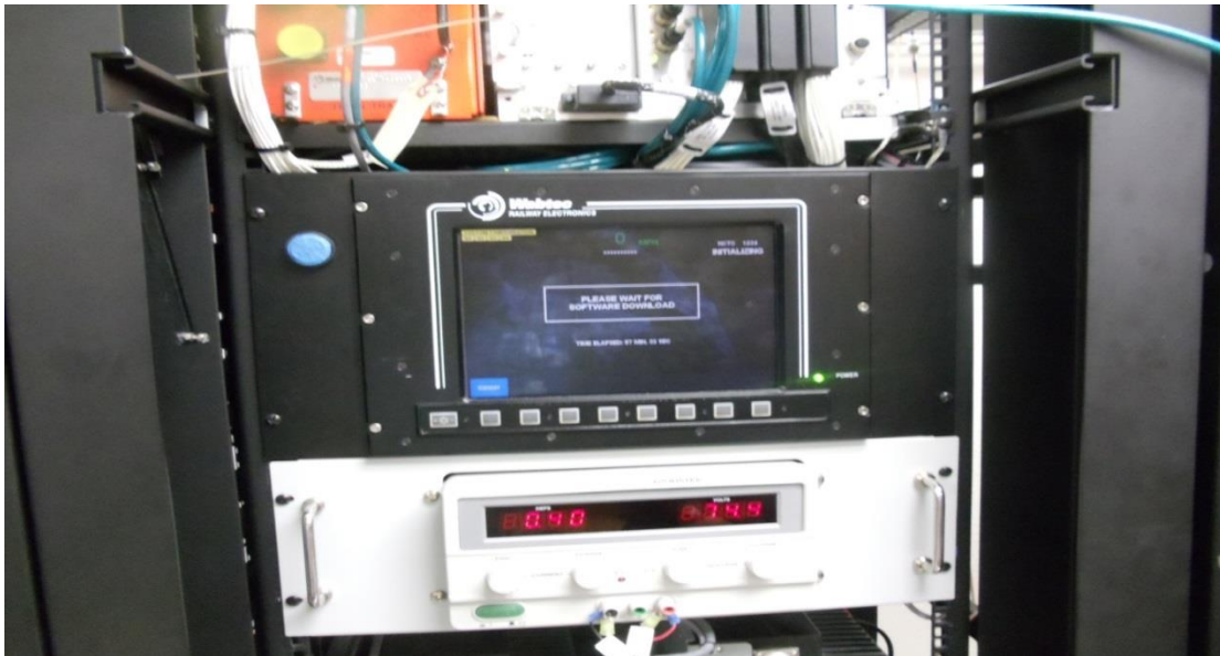
NCTD continues to make slow progress in their implementation of PTC. The new goal is to have PTC operational by the end of the year.
