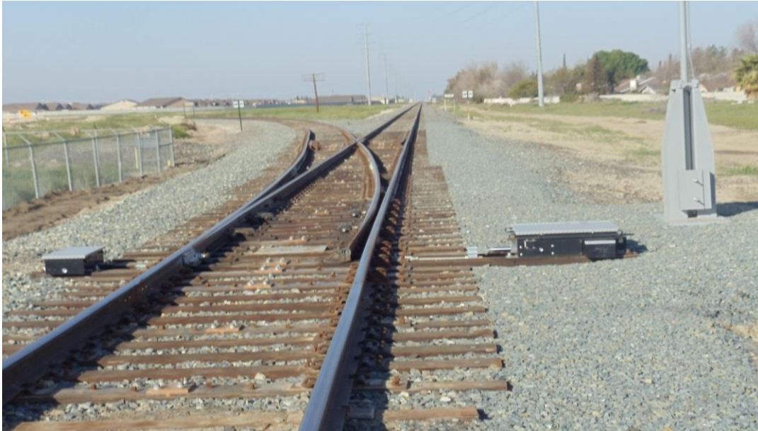
Radio controlled switch on the Buttonwillow subdivision, Kern County
