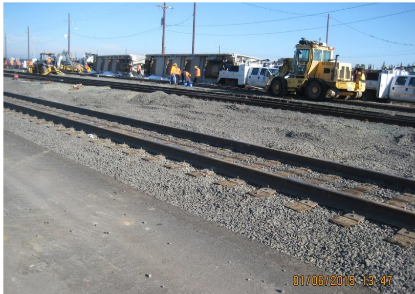
Derailement site with UP's track gang working to restore track
