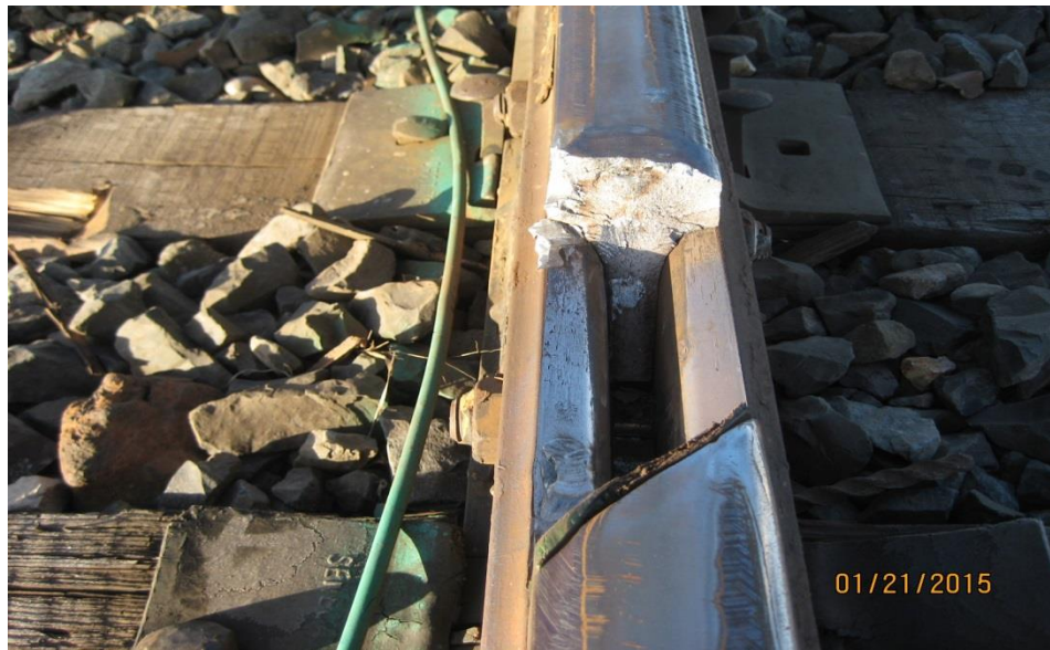
View of discovered breakout in rail as a result of a bolt-hole crack at a miter cut insulated joint
