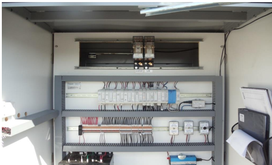
Picture of inside of control case.
