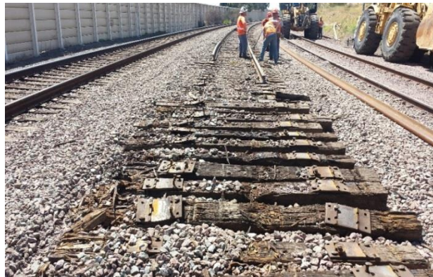
Derailed site illustrating track damage at Esperanza.
