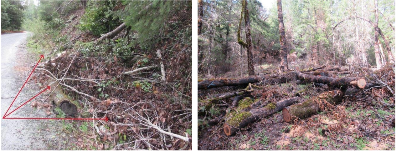
Figure 20: Inspection Area A: Wood Management "debris in road drainage" non-compliant (left). PIIR site with non-compliant Wood Management (right)
