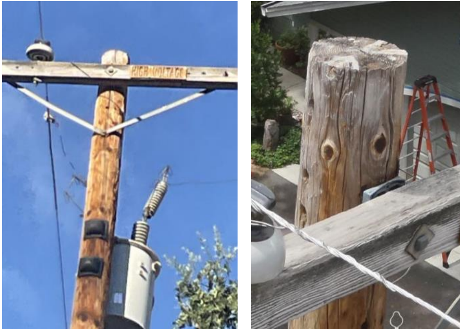
Figure 16: Aerial Cancellation of Ground Finding E Tag
