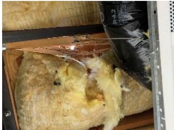
Figure 23. Navigation Center roof hole caused by debris.
