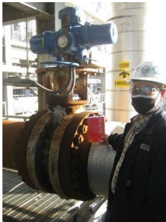
Figure 31. The Cold Reheat Valve that allowed the accumulated water to enter the Steam turbine.
