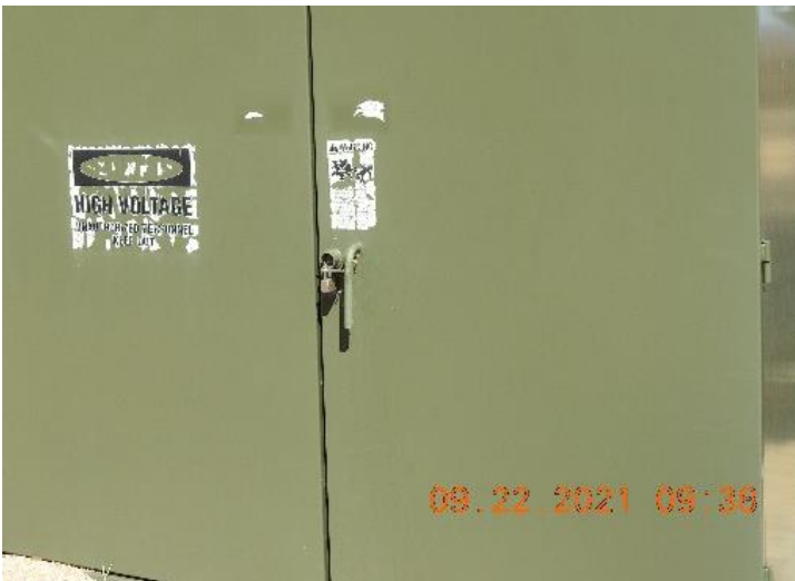
Several deteriorated high voltage stickers on outdoor transformers.
