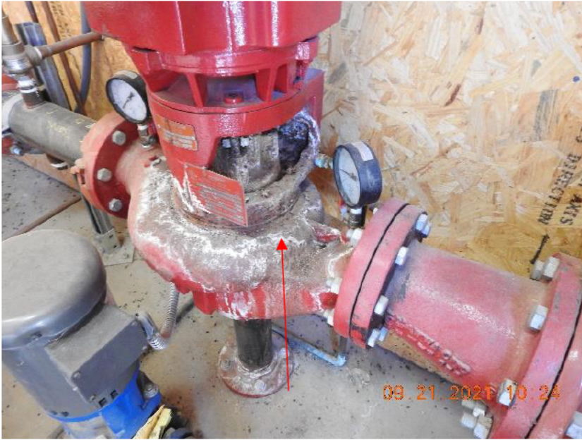
Buildup around fire pump suggests water leakage over a long period of time.
