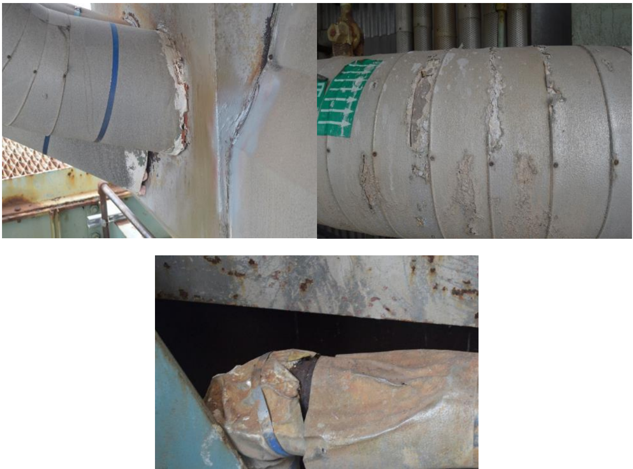
Figure 1: Damaged insulation around the Plant
