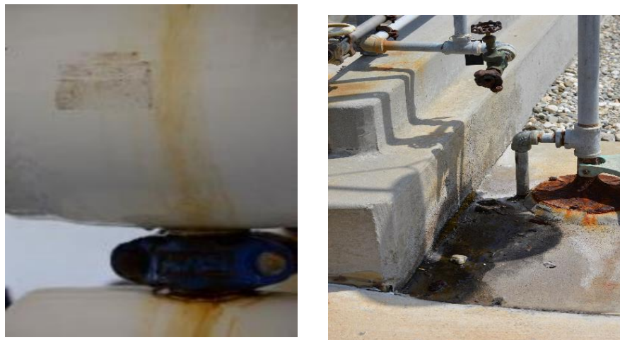
Figure 3: Minor leak in RO truck (left) and another minor leak (right)
