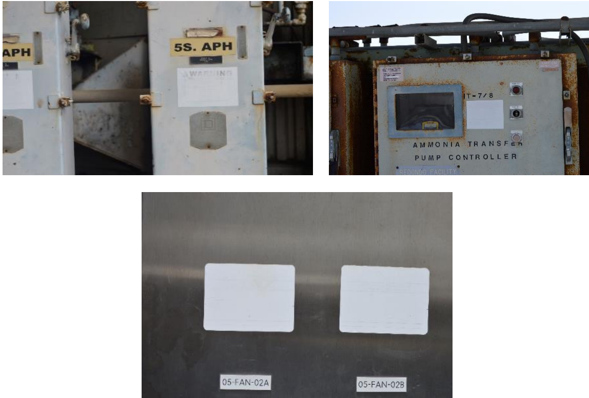
Figure 10: Missing Arc Flash Stickers
