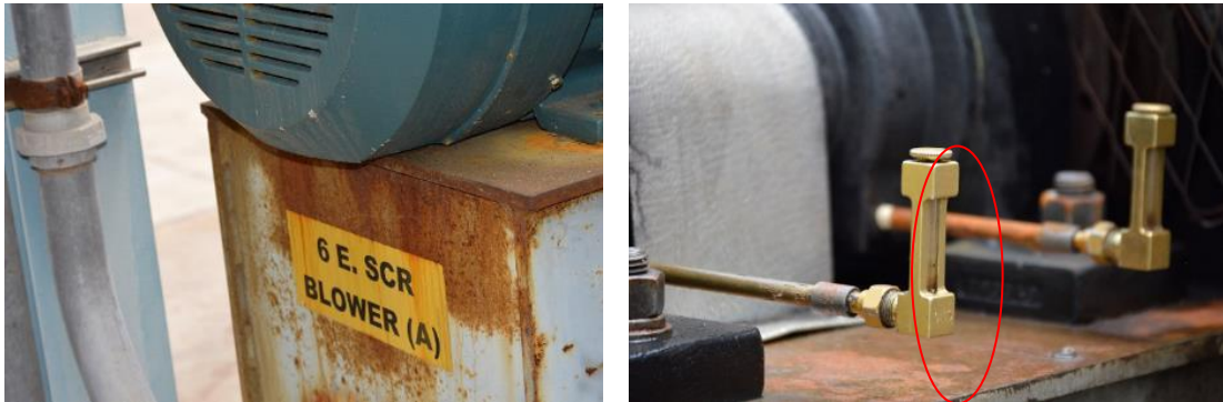
Figure 2: Low lube oil level in 6 E. SCR Blower (A)
