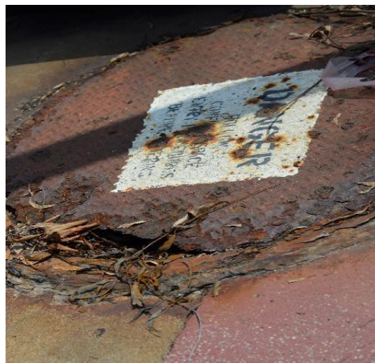
Figure 8: Corroded and damaged Confined Space cover
