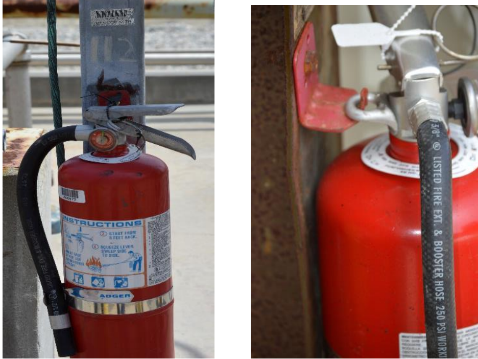
Figure 13: Fire extinguishers with missing current annual inspection tags.
