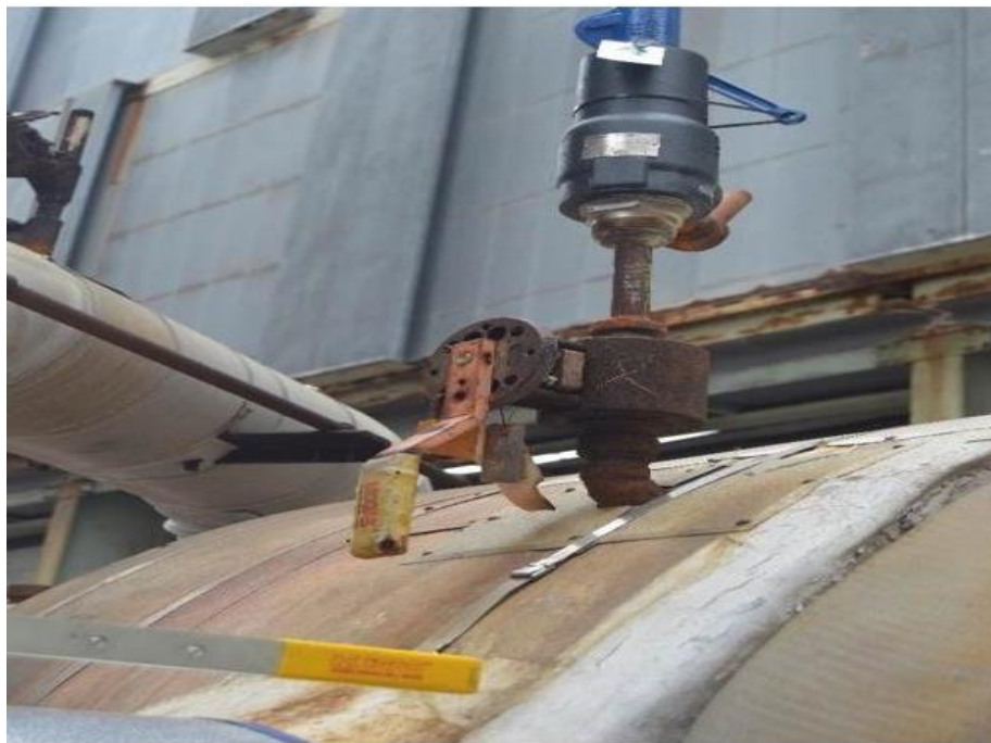
Figure 15: Stop valves installed at upstream of relief valves on heat exchangers
