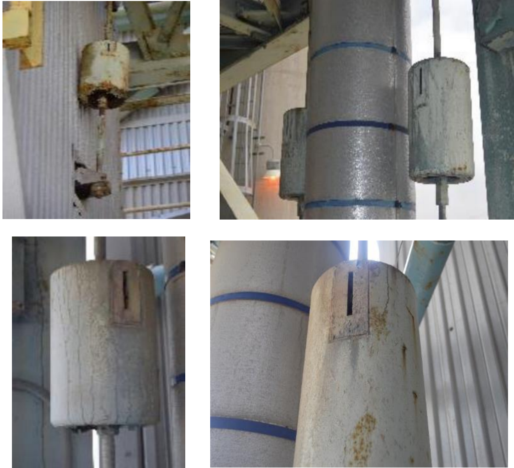
Figure 14: Unmarked HEP supports
