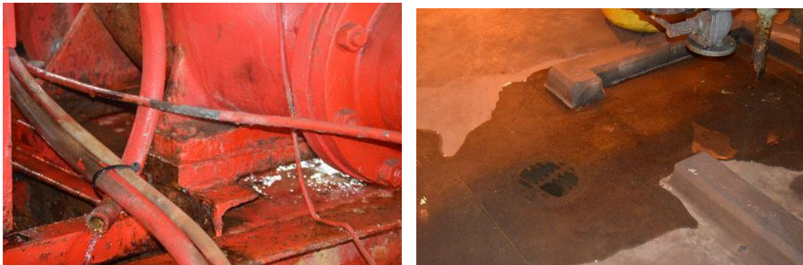
Figure 5: Drain line not properly tied to drain (Left) and a clogged drain resulting in standing water (Right)
