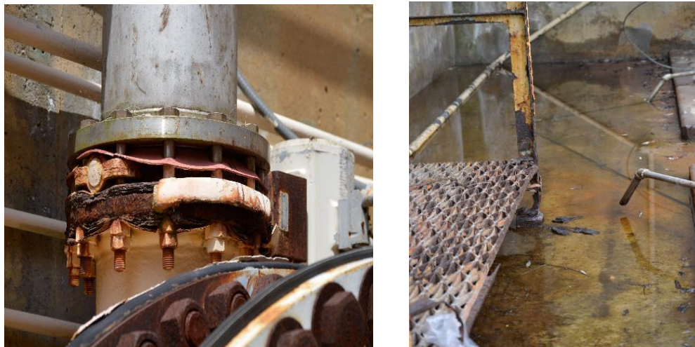
Figure 12: Corrosion in flange (left) and standing water (right)
