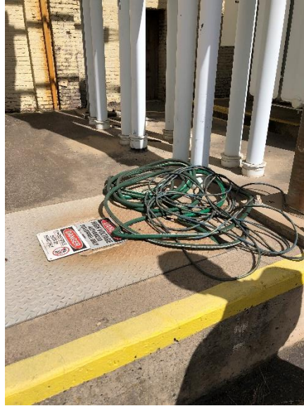
Figure 12. A water hose and a cord on top of a confined space entrance.
