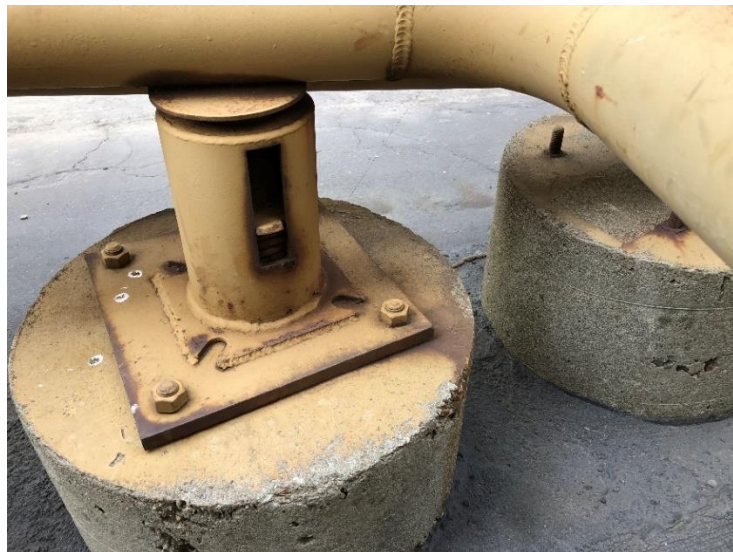
Figure 6. A fully compressed spring-loaded pipe support.
