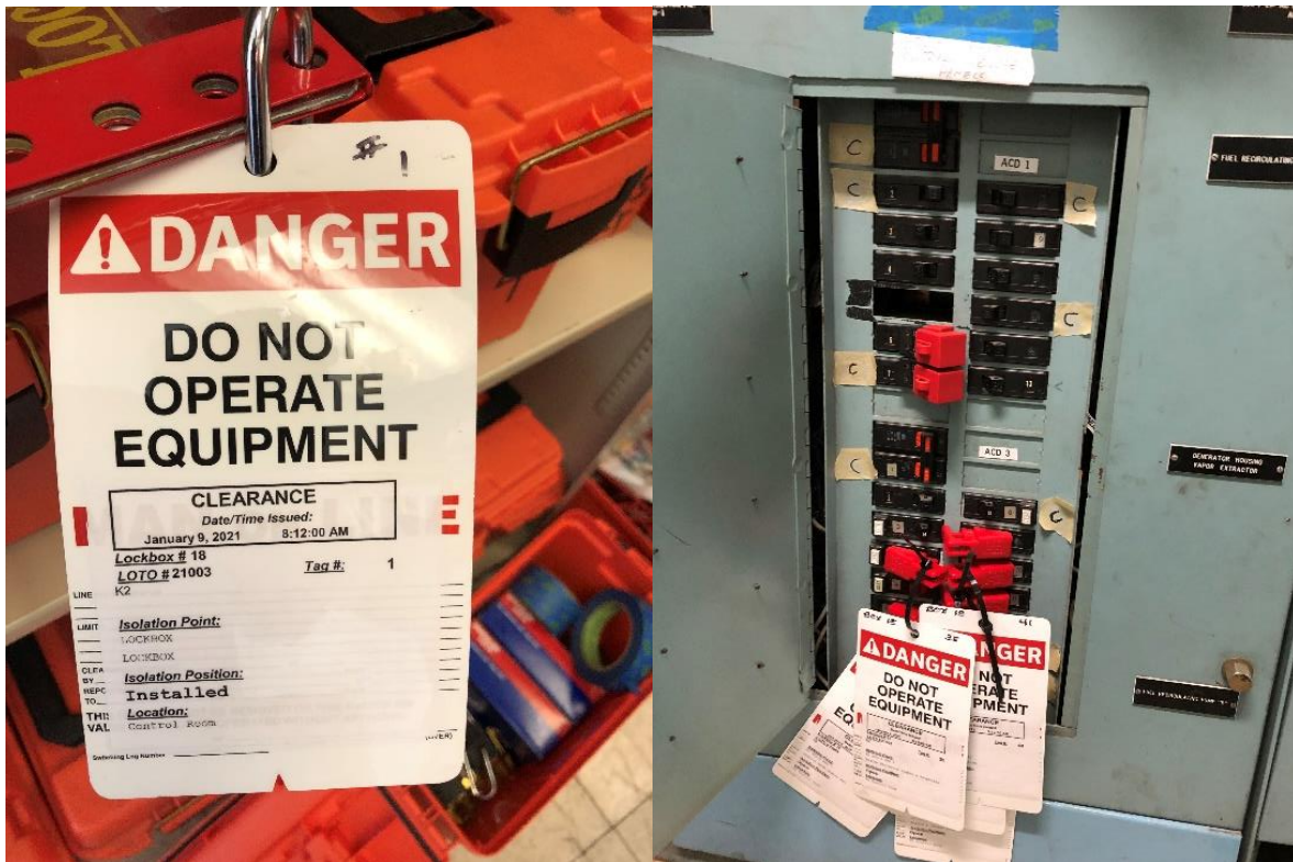
Figure 4. LOTO #21003 Tag #1 at the lock box (Left photo). The circuit breaker box that is missing LOTO tags (Right photo).
