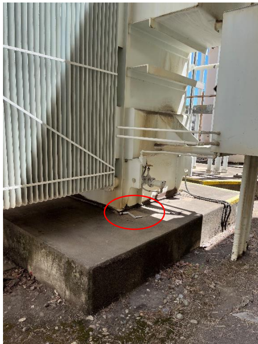
Figure 11. A hand crank on the concrete pedestal at Transformer #7.
