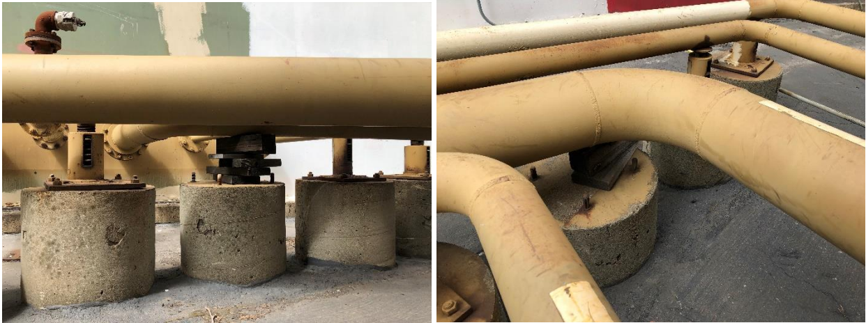
Figure 5. Two locations where the spring-loaded pipe supports have been replaced with stacks of wood.
