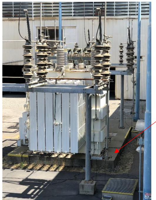
Figure 7. Transformer #9 for Unit K3, with the arrow pointing to the air switch handle.
