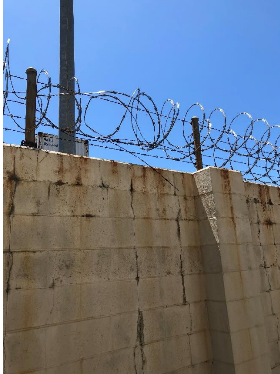
Figure 9. Broken barb wire along the western perimeter wall.
