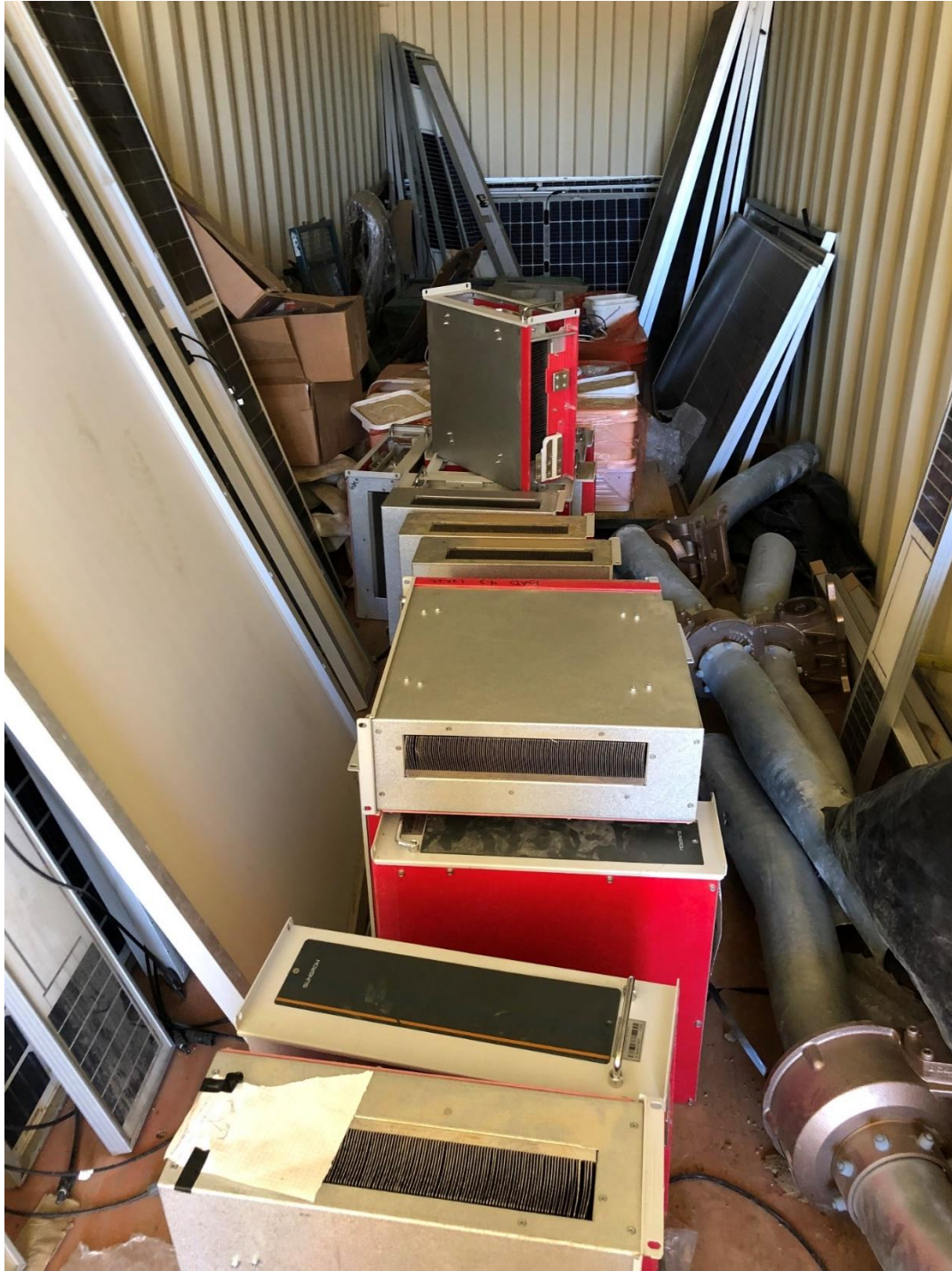
Figure 3: Equipment improperly stored inside storage container
