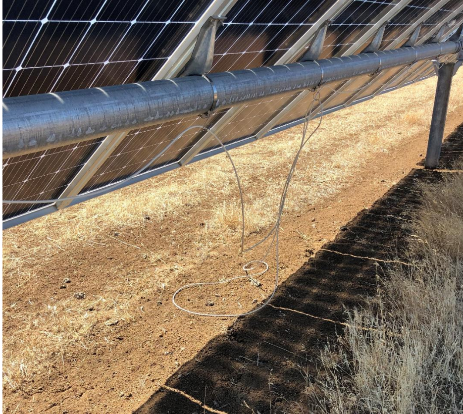
Figure 6: Showing conductors on an array 1 row East of CB1.9.1C9
