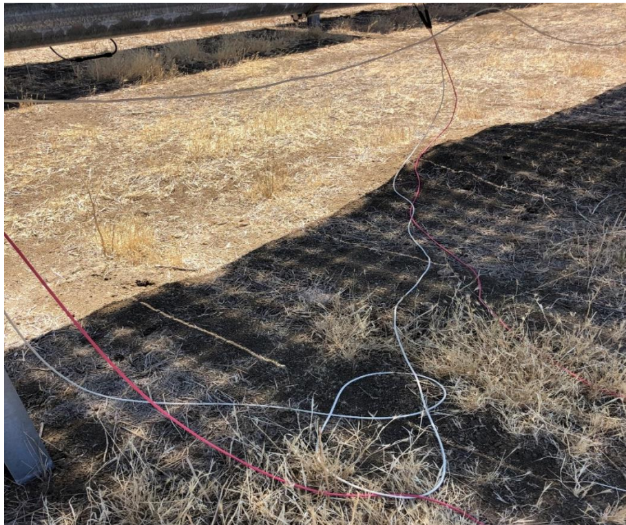
Figure 8: Showing conductors on an array near CB 1.16.5C13.
