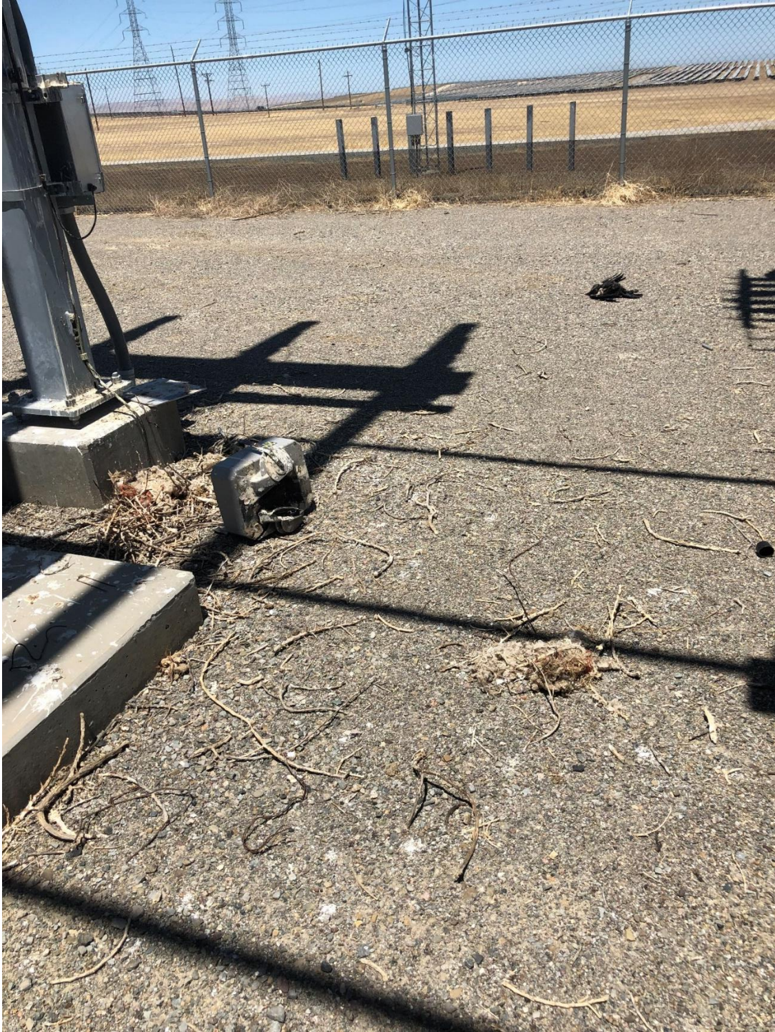
Figure 1: Showing remains of a bird strike left in the substation.
