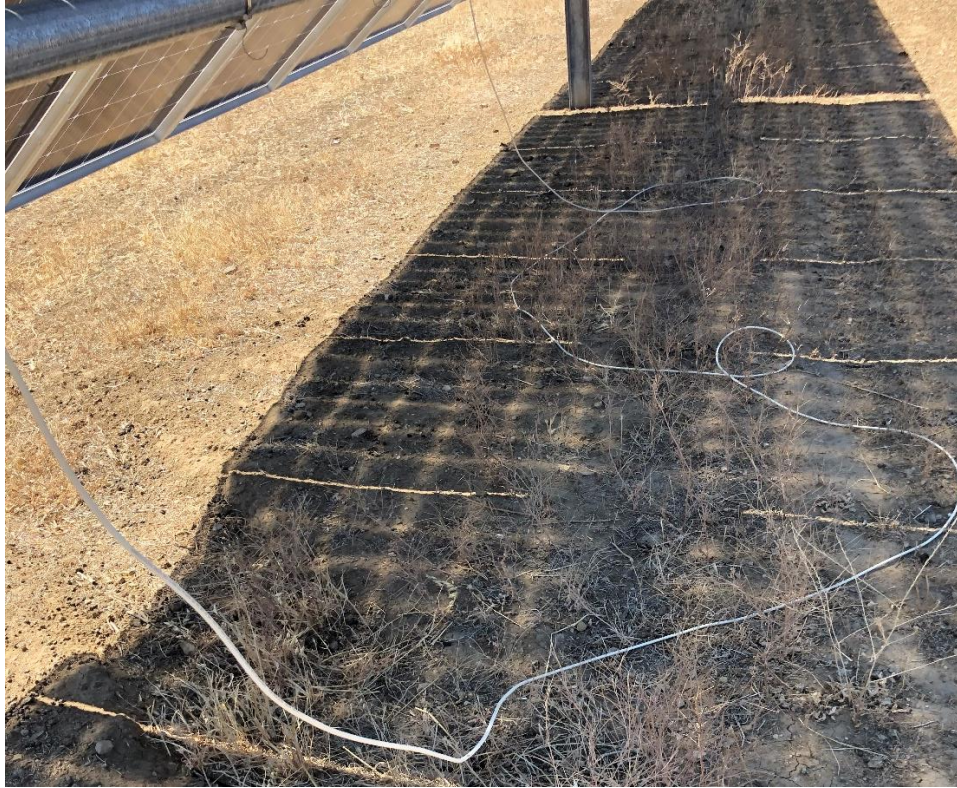
Figure 7: Showing conductors on an array near CB1.9.1C10
