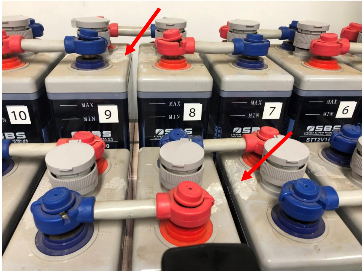
Figure 2: Chemical build-up on the substation battery bank
