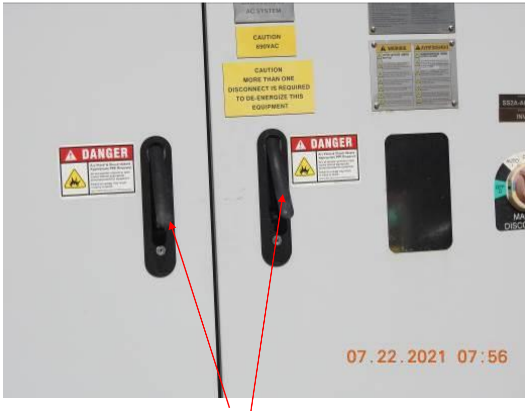
Broken Door handles, some doors were not locked properly
