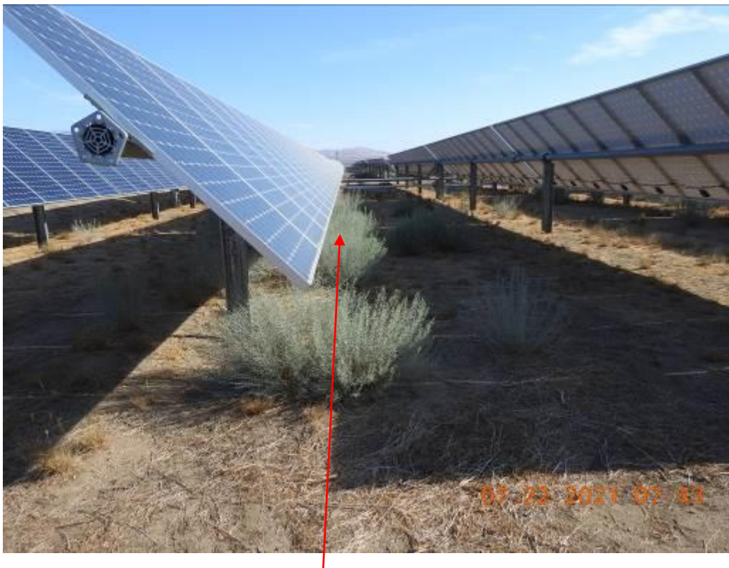
Vegetation near solar panel
