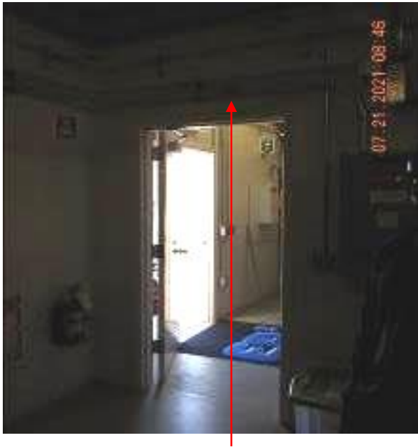
No Exit sign
