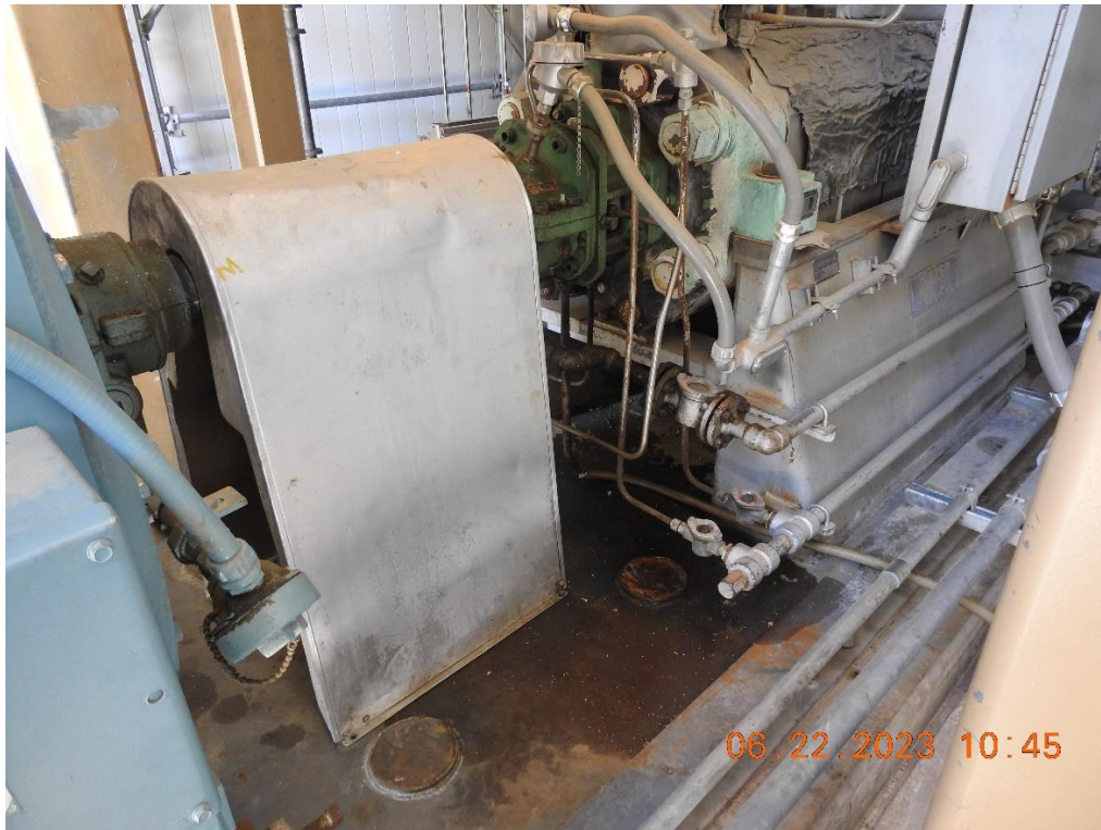
Figure 1: Oil leak from Unit 2 boiler feedwater pump.
