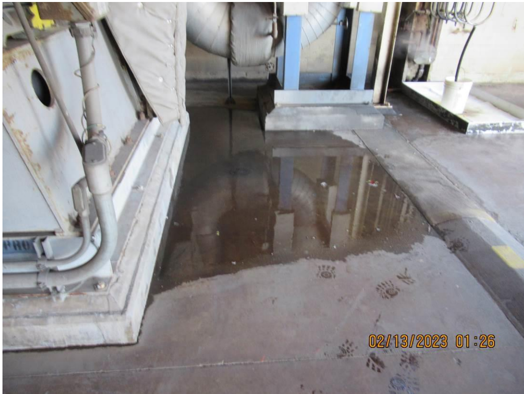
Figure 1: Standing water because of clogged drain
