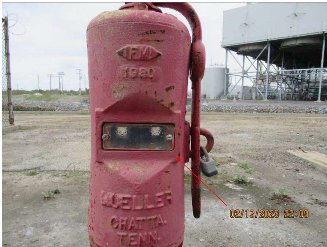
Figure 13: PIV missing position indicator
