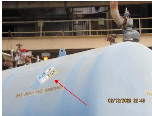
Figure 6: Damaged NFPA sign (fire diamond)
