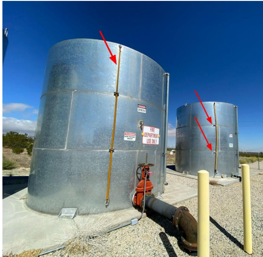
Figure 4: (Left) Yellowing fire water level indicator pipe. (Right) Unsecured and yellowed potable water level indicator pipe.
