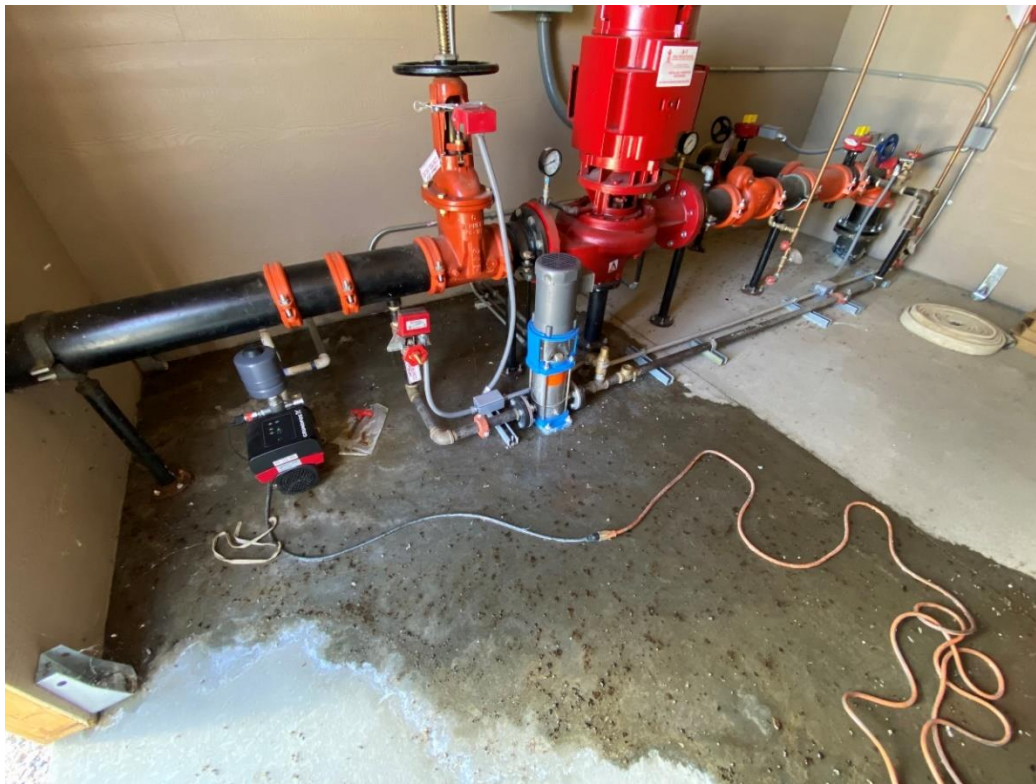
Figure 3 : Energized extension cord plug lying in standing water.
