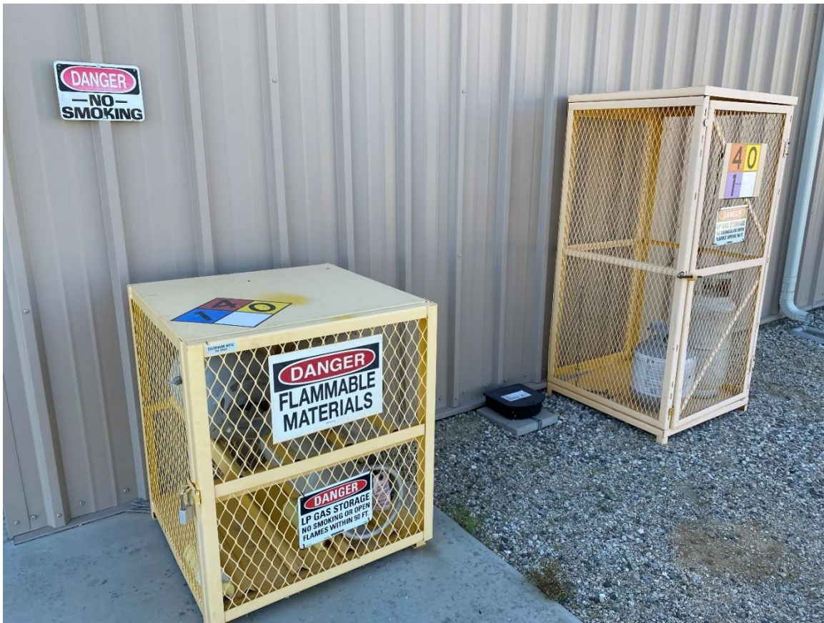
Figure 2: Incorrect NFPA 704 diamonds on the liquid propane gas storage tanks.
