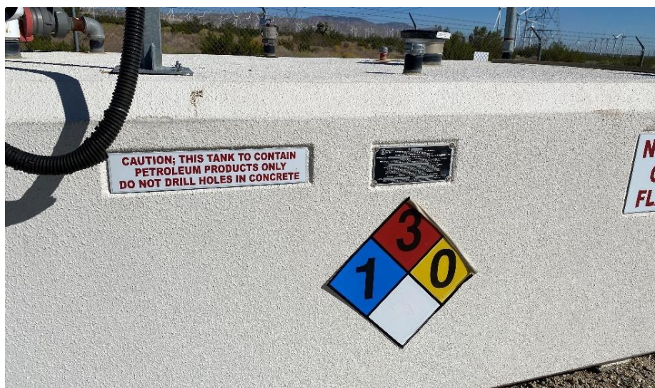
Figure 1: Incorrect NFPA 704 diamond on the unleaded gasoline storage tank.
