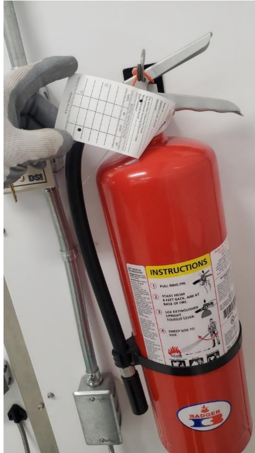
Figure 6: Fire extinguisher in the substation building is missing monthly inspection sign offs.
