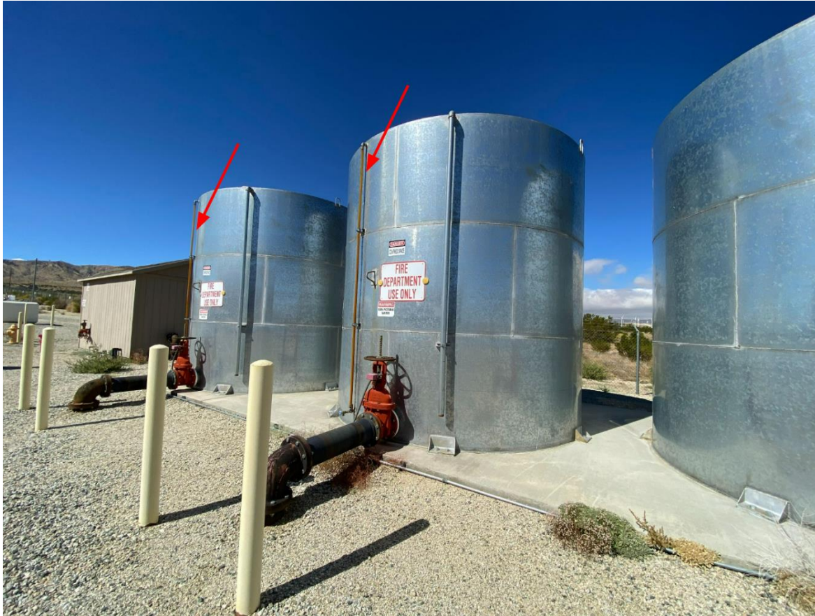
Figure 5: The fire water level indicator pipes are yellowed and opaque.
