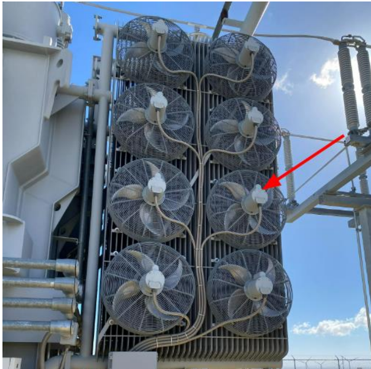
Figure 9: One GSU fan was not operating during the manual fan test.
