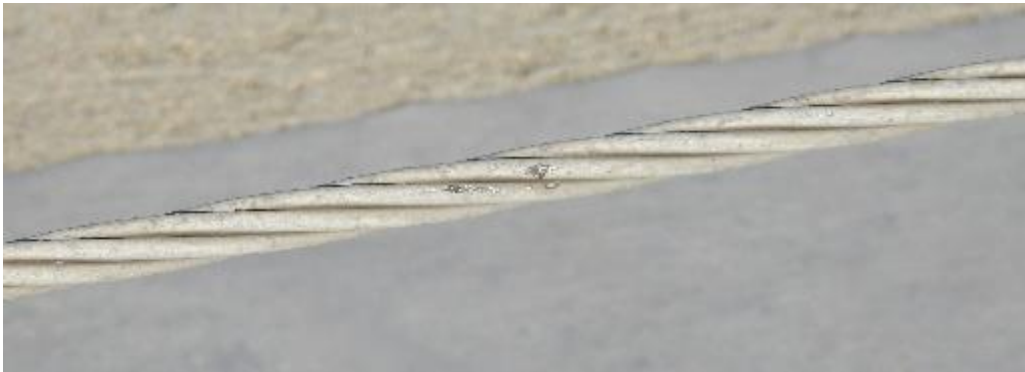
Figure 6: Damage at 154 feet along SCE's middle conductor
