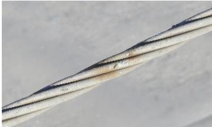
Figure 5: Damage at 196 feet on SCE's southmost conductor
