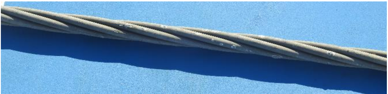
Figure 3: Damage at 169 feet on SCE’s southmost conductor
