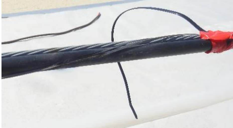
Figure 7: Additional damage near where the third lashing wire parted
