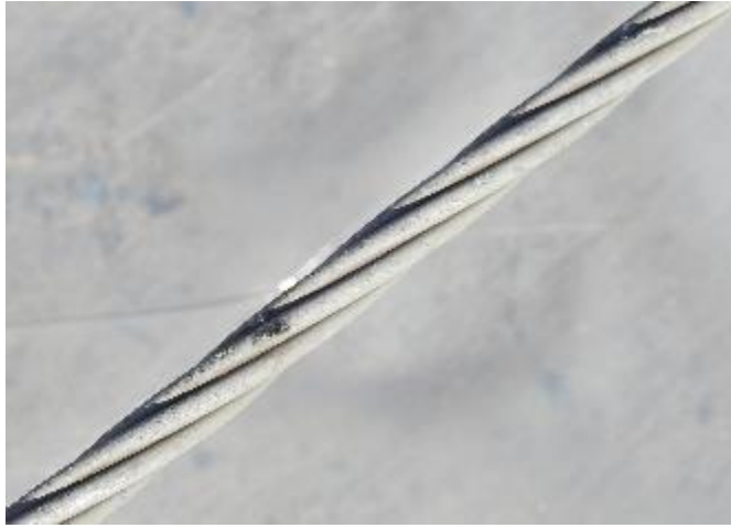
Figure 4: Damage at 196 feet on SCE's southmost conductor
