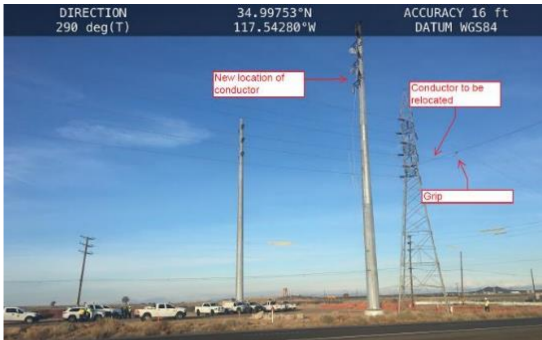
Figure 3: The scene of the incident on the day it occurred. The bucket truck was near the steel lattice tower. Although the conductors were bonded together here, none of the structures in this photograph were grounded.
