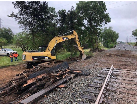
Debris from bridge demolished after fire
