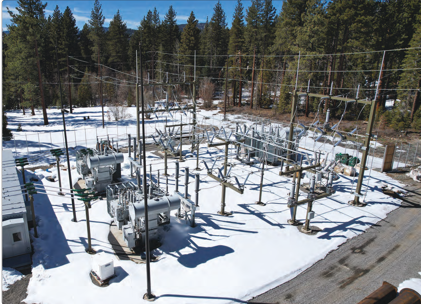
A Liberty Utilities CalPECO Lake Tahoe Substation
