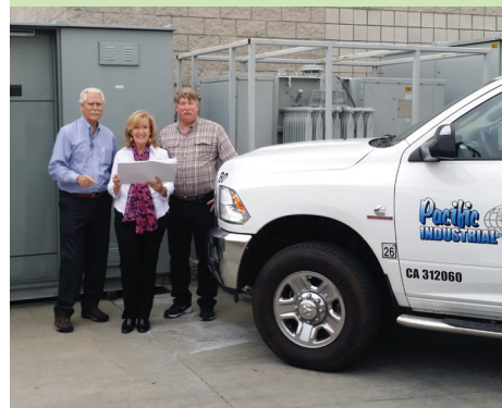
Hired by SoCalGas, the Pacific Industrial Electric team worked on a project to reduce carbon emissions from San Nicolas Island.
