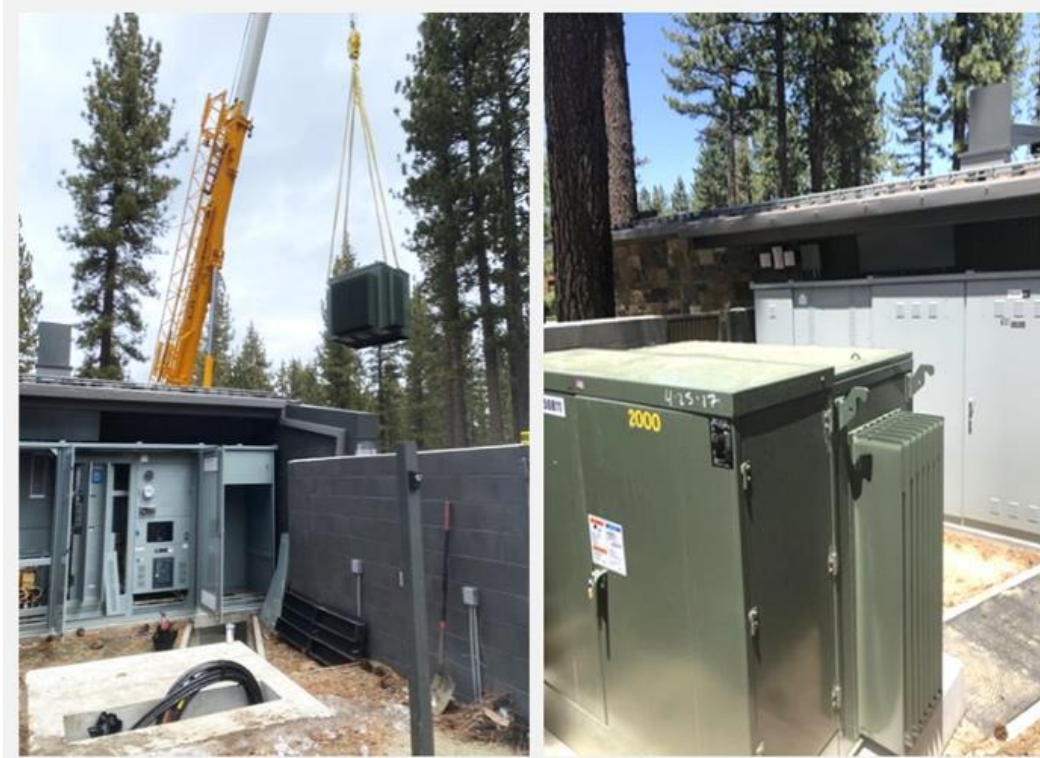
Crane installing transformer behind bus stop (left) and the installed transformer and switchgear (right)
