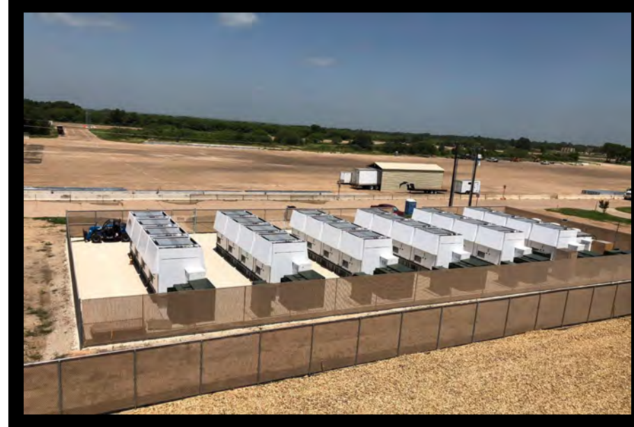
Texas A&M RELLIS, 2017 10.5 MW Natural Gas
