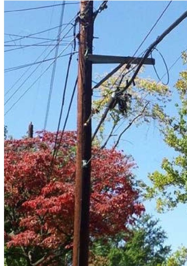
Figure 10: Example of extension arm on pole, enabling horizontal expansion of capacity
